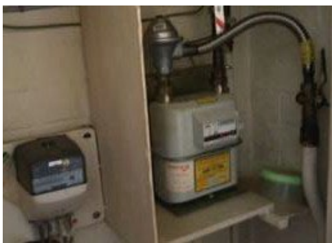
Asbestos panelling around a gas meter
