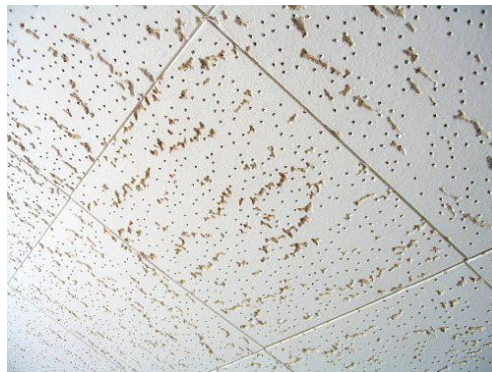
Asbestos containing ceiling tiles
