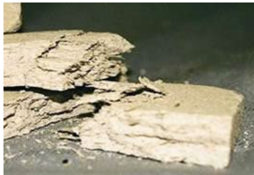
Pieces of Asbestos Insulating Board (AIB)
