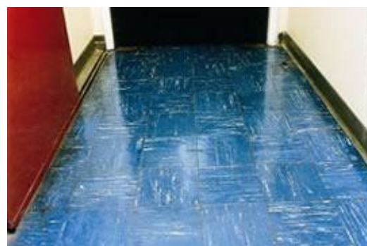
Asbestos containing floor tiles in a corridor
