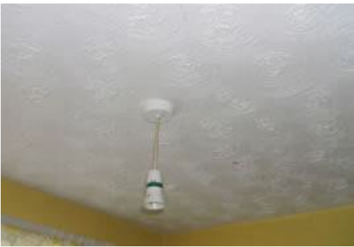
Asbestos textured coating
